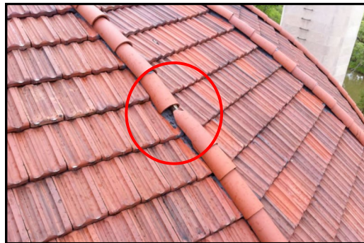
damaged tile on dome roof
