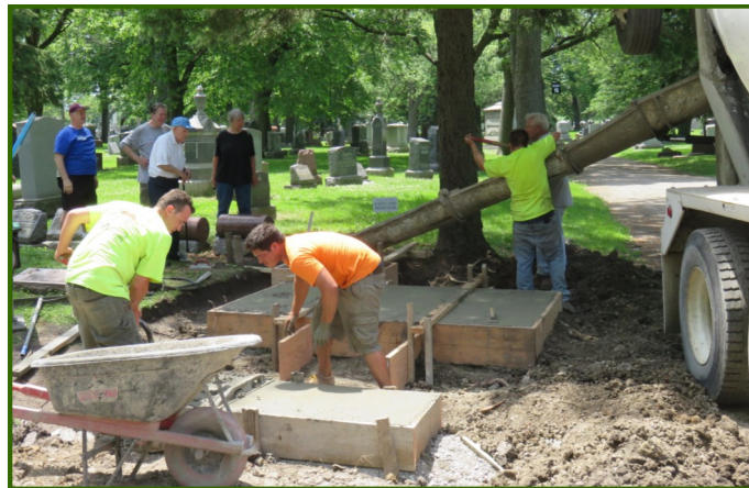
Pouring of the foundations for the Eastland Memorial that will be dedicated on July 12. See page 5 for more information.
