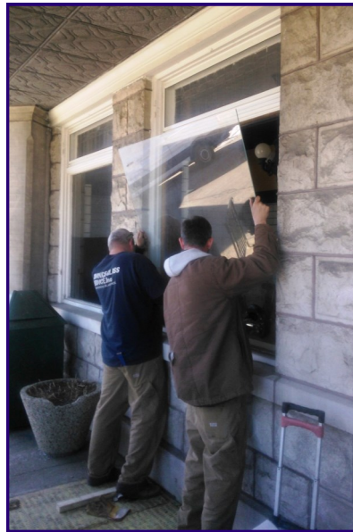
A new window is installed in the gatehouse, paid for by Friends of BNC. (photo by Chuck Michalek)
